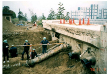
SUPER FLEX on bridge abutment in Kobe area had no damage during Kobe earthquake in 1995. (Measured subsidence : 1100MM)
